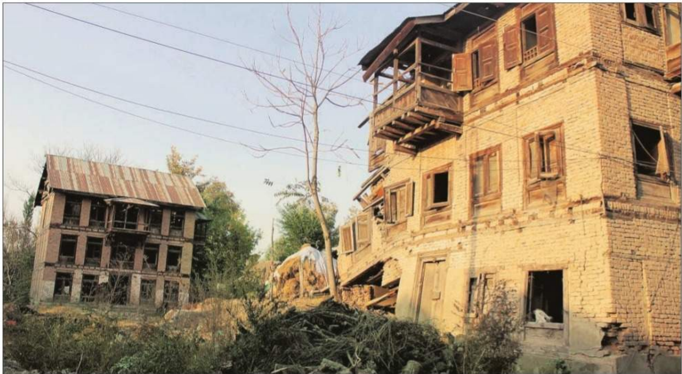
In Simroo village of Pulwama, the once majestic mud-and-brick houses owned by Kashmiri Pandits are now crumbling. October 2016 file picture by Sofi Ahsan
