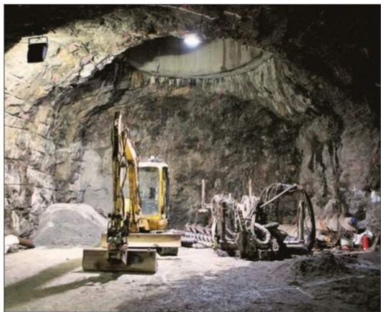
Excavating equipment at the site of what will be the world's first repository for spent nuclear reactor fuel, deep in granite bedrock in Finland. Miikka Pirinen for The New York Times
